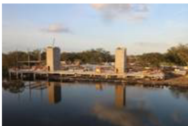
Construction site for the new $45.5MM Louisiana Children's Museum in New Orleans City Park.
